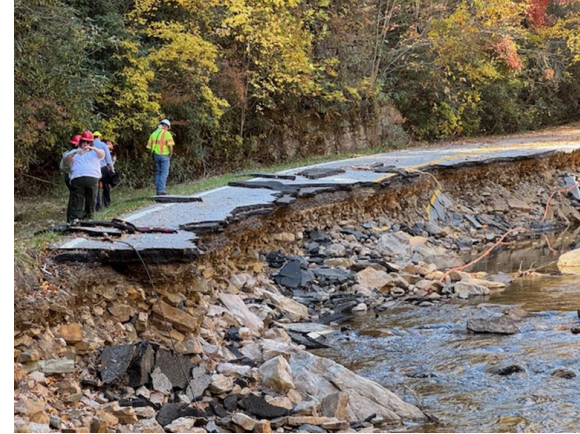
Over a mile of Route 58 destroyed
